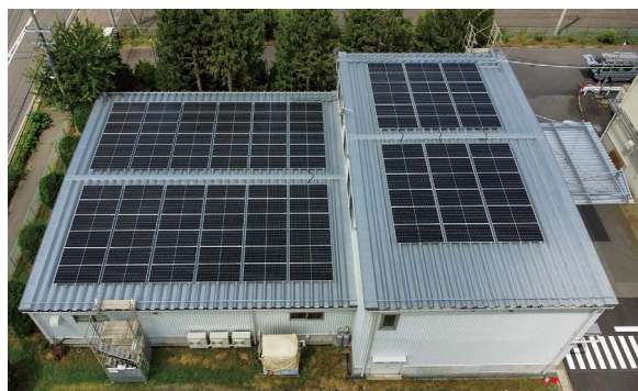
A solar power generation system was installed at the Matsumoto office of Kawai Seimitsu Kinzoku Co., Ltd.
